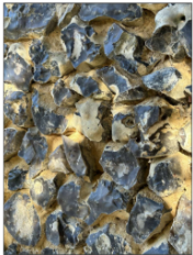
04 Boundary Wall - Loose Flints NTS
