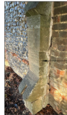
05 Boundary Wall - Damaged Pier NTS
