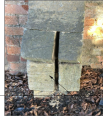
03 Boundary Wall - Damaged Pier Base NTS
