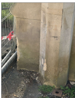
03 Damage to Gate Opening Reveal NTS
