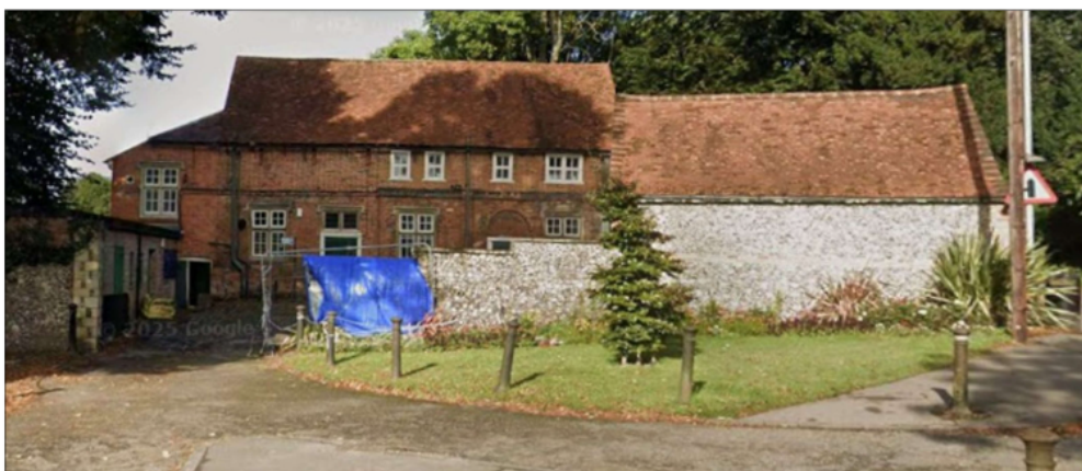
02 Stable Block Gateway & Piers Showing Damage from Highway NTS
